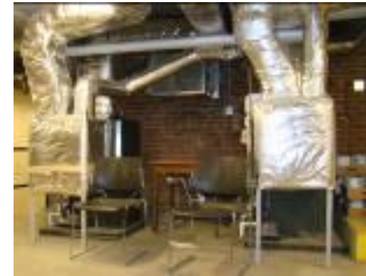
Water to air heat pumps
