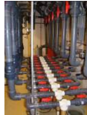
Piping and valves
